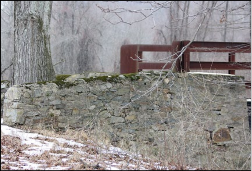
The original stonework is still visible – and in use – at the Scott's Mill Bridge.
